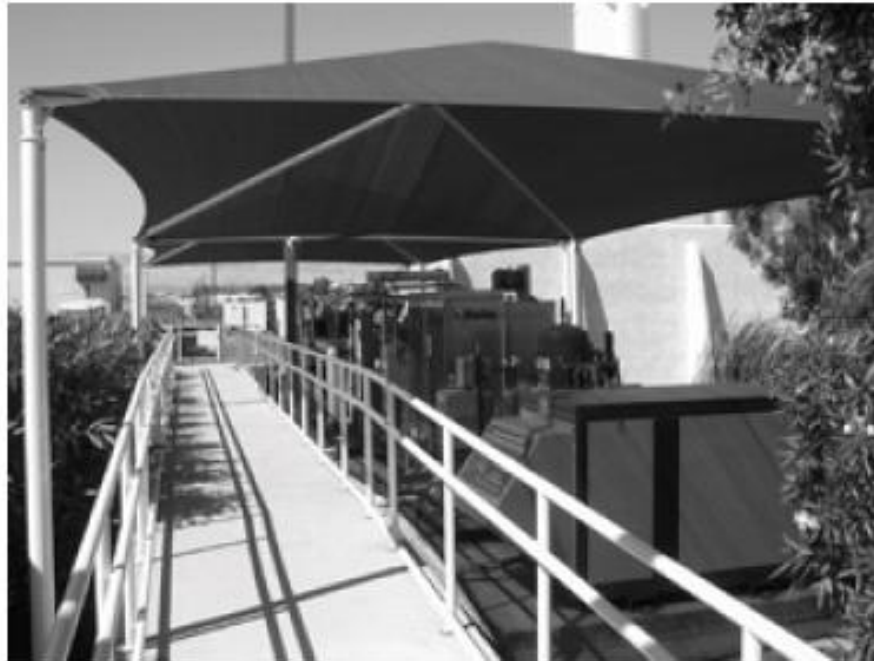
HbT's Model 4200 NG-A natural gas reformer system at SunLine Transit Agency
