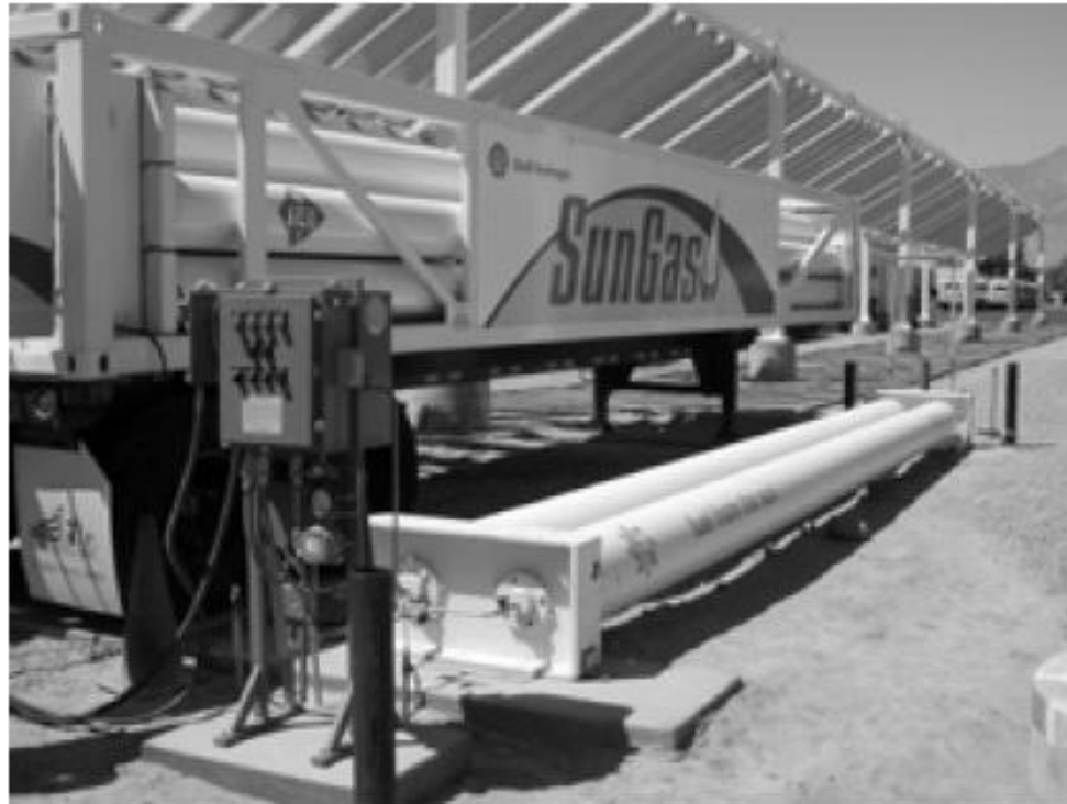
SunLine's FIBA tube trailer and ASME tanks for CH 2 storage
